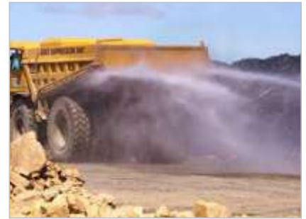
Pump for Dust Suppression System
