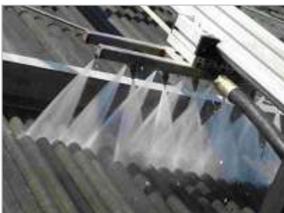
Pump for ACC Fin Tube Cleaning
